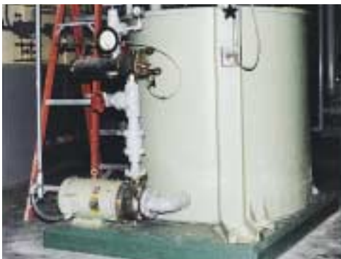
Reverse osmosis, Ósmosis invertida
